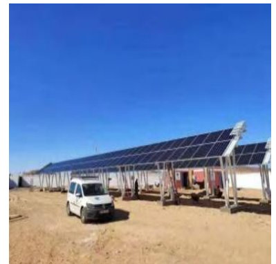
500KW Project in Panama
