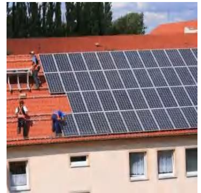
40KW Project in Malaysia
