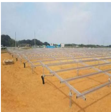
4MW Project in Mysore
