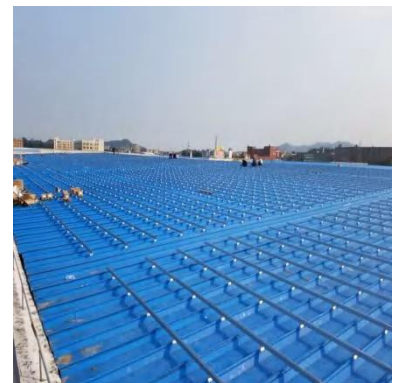
4MW Project in Vietnam
